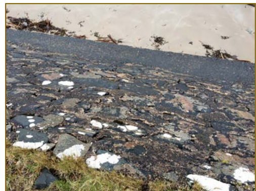
7. BULGING AND VOIDED STONEWORK
