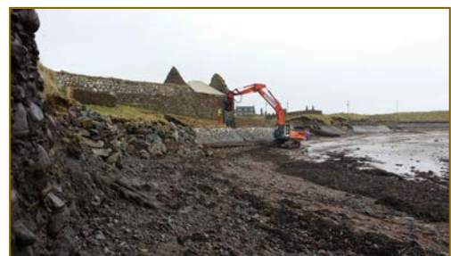
6. LANDSLIP IN THE EAST PART OF THE REVETMENT.
