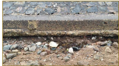
5. UNDERMINED CONCRETE TOE, ALSO VISIBLE VOIDS IN THE STONEWORK
