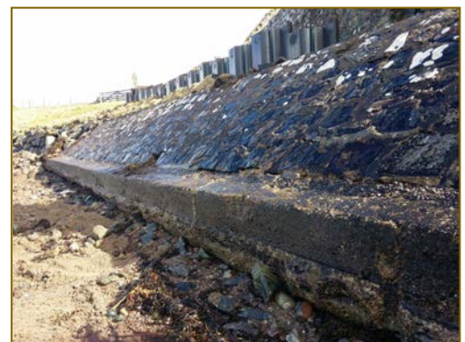
4. ANOTHER VIEW ON THE UNDERMINED TOE AND VOIDED AND BULGING ARMOUR STONE REVETMENT
