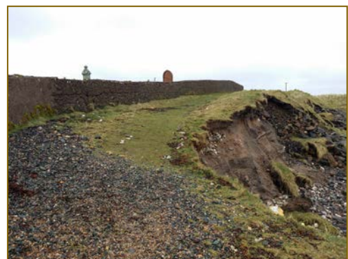
8. SEVERE LOSS OF GROUND WEST OF THE CHURCH CAUSING SERIOUS PUBLIC SAFETY ISSUE; ALSO THIS IS AREA OF OUTSTANDING ARCHAEOLOGICAL IMPORTANCE
