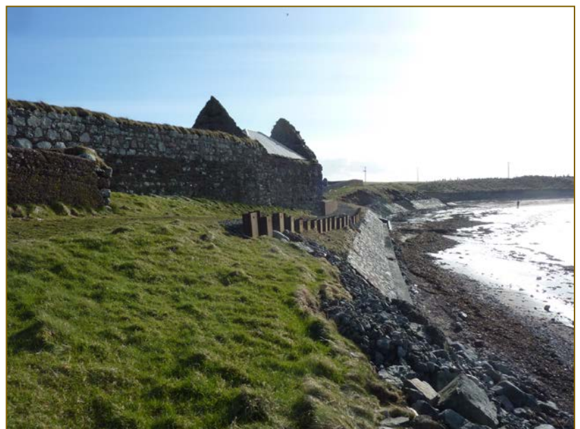
10. OVERALL VIEW OF THE COASTLINE SHOWING ALL THE AREAS OF DAMAGE
