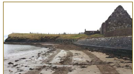
3. VIEW ON UNDERMINED CONCRETE TOE OF THE REVETMENT ALONG THE CHURCH AND LANDSLIP
