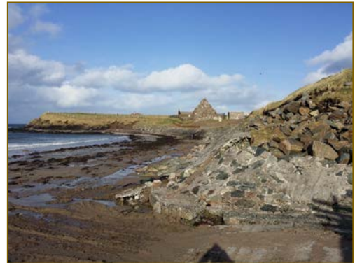
9. DAMAGE TO SIDE OF SLEEPWAY
