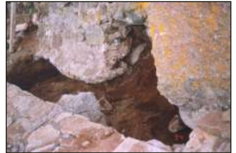
BLOW HOLE UNDER THE FOUNDATION OF WEST CHAPEL
